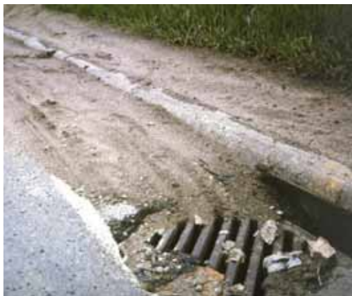
Sediment entering a storm sewer inlet as a result of construction related erosion.
